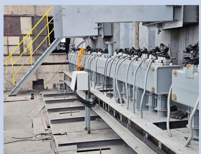
Clay filter purging system
