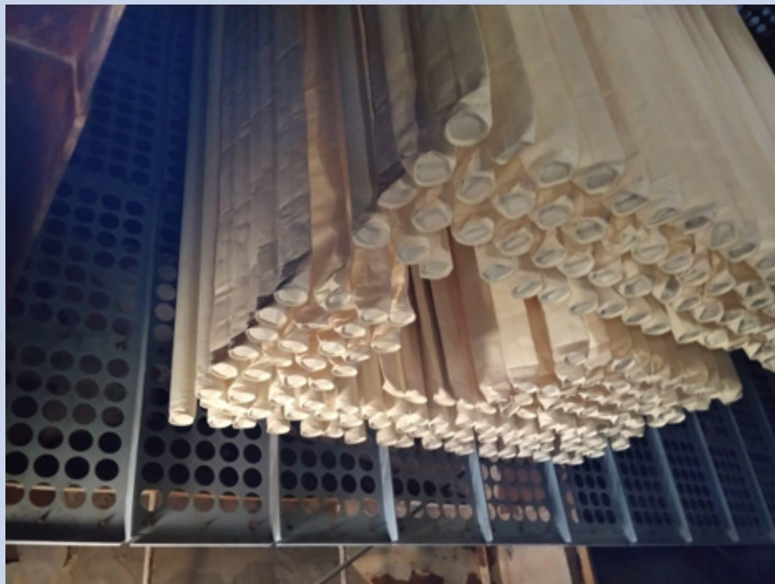
New bag filter for clay chamber.
